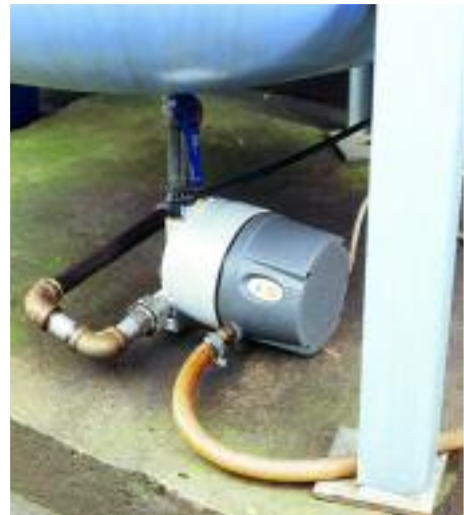
ED2300 installed on an air receiver.
