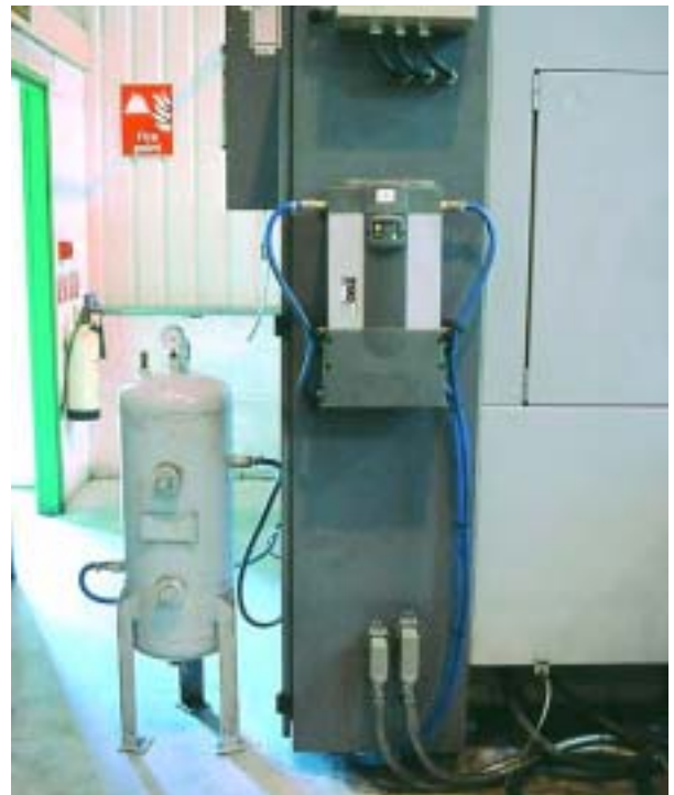
PNEUDRI MiDAS installed to supply control air for a CNC machining centre
