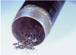
Corrosion of piping
